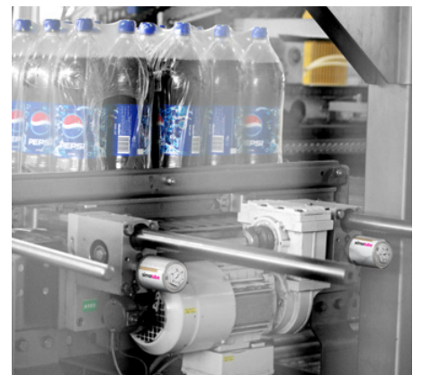
The bearing on the gear box is lubricated with two 60 ml simalube lubricators.
