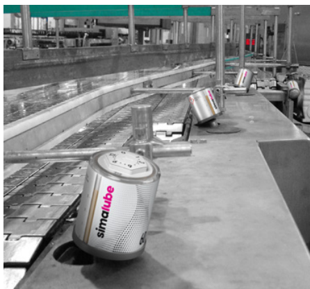
A filling line is equipped with several simalube lubricators.
